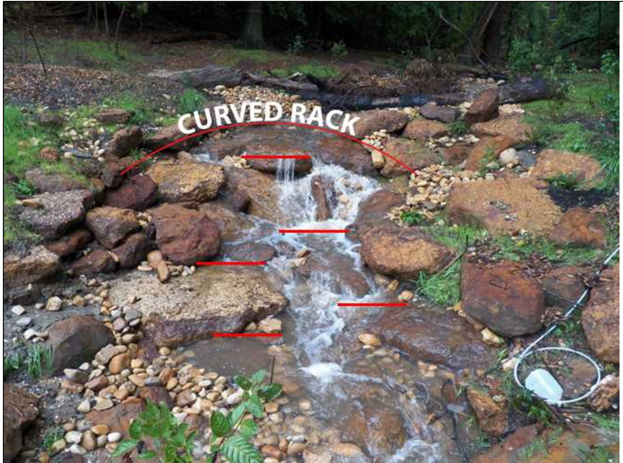
Figure 53. Gentle curved rack spreads flow across the cascade. Flat and alternating placement of boulders breaks flow. Tie in boulders extend into the berm or existing ground with many buried.
