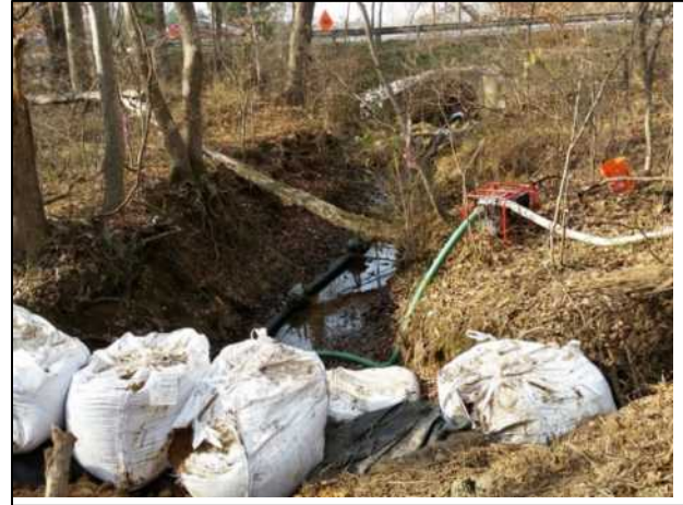
Figure 25. Slotted pipe underdrain must be used in conjunction with a pump around practice that is sized to handle the volumes of the drainage area.
