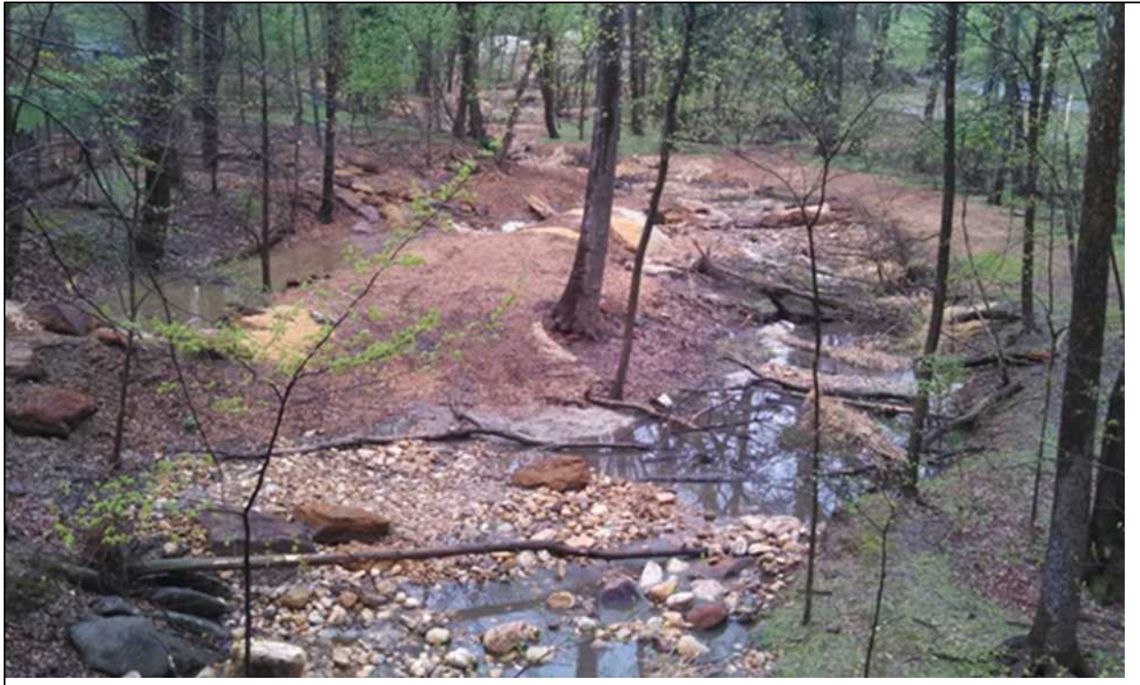
Figure 15. Both larger and smaller trees are left in place during the construction of the haul road and iteratively removed or incorporated into the project during weir and pool construction. Trees removed during construction are used as coarse woody debris in addition to imported stumps, logs and branches.
