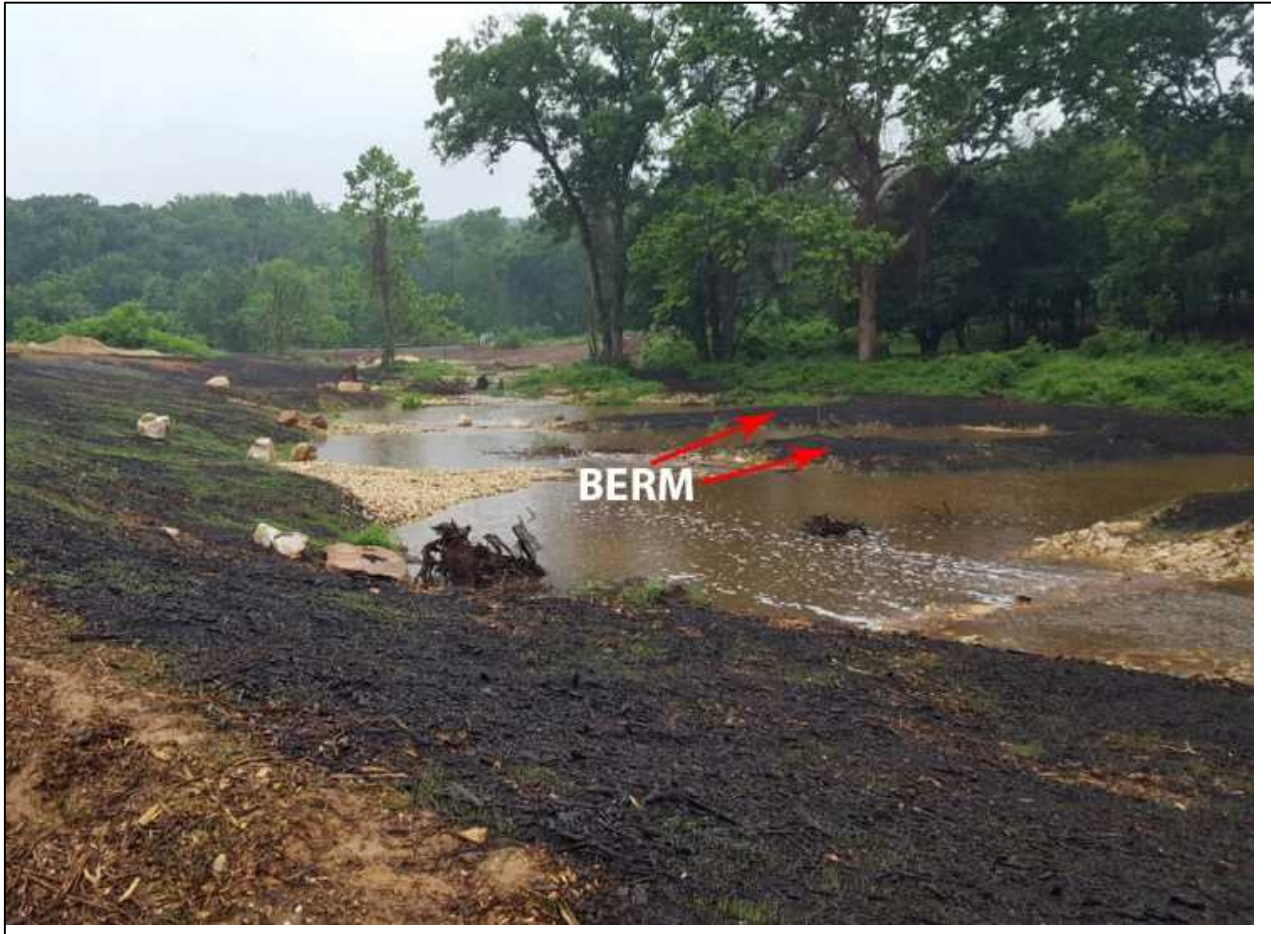
Figure 45. Berms holding water to keep flow from cutting around the weir, spreading water out, increasing exchanges of surface and groundwater and filtering water through their medium.
