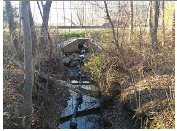
Figure 22. Slotted pipe is inserted into outfall and capped. For large drainage areas, sandbag dikes should be installed sufficiently downstream to create pooling area, as seen in the photo, for clean water diversion.
