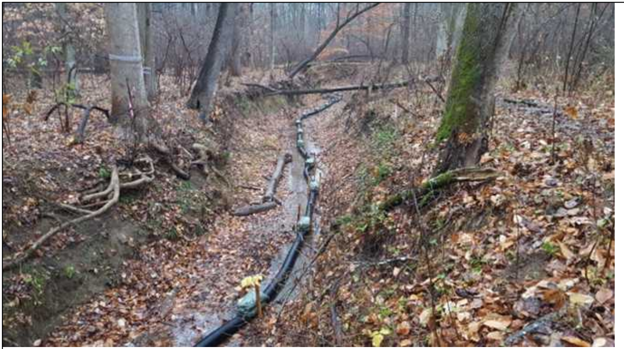
Figure 20. Slotted underdrain system functions as a french drain to help keep haul road dry and convey baseflow during construction. Sections of pipe must be removed during sequential construction of pools to restore surface flow.
