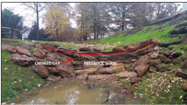
Figure 51. Subgrade is excavated to support a parabolic shape necessary to keep flow in the center and shoulders. Boulders are placed flat to create falls from top boulder to next rather than continuous surface in a chute. Gaps between boulders have been filled by hand-placing smaller boulders and rock (chinking) in a manner that maintains the general line of the boulders. Range of gravel and cobble sizes have been randomly cast throughout the cascade to allow self-organization throughout time. Spaces between boulders are planted and seed is cast over entire structure to stabilize and naturalize over time.
