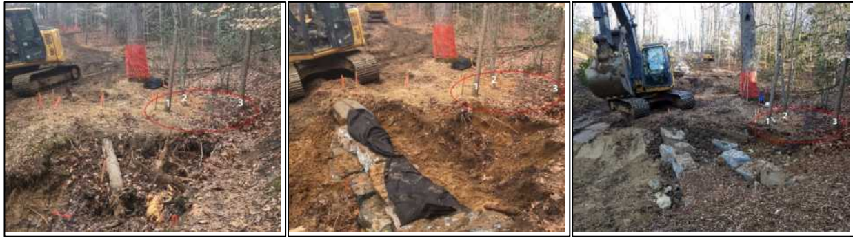
Figure 36. Large trees voluntarily marked with orange construction fencing to avoid removal before haul road construction. Smaller trees saved by the contractor until weir construction before determining need for removal. The contractor successfully constructed the weir per plans without removing the trees (red circles show same trees pre, during and post construction).
