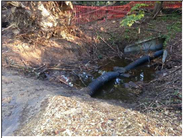
Figure 21. Slotted pipe is inserted into pipe and capped. For smaller drainage areas, haul road can begin immediately downstream as seen in the bottom left of photo. Small pumps can be used to dewater if necessary.
