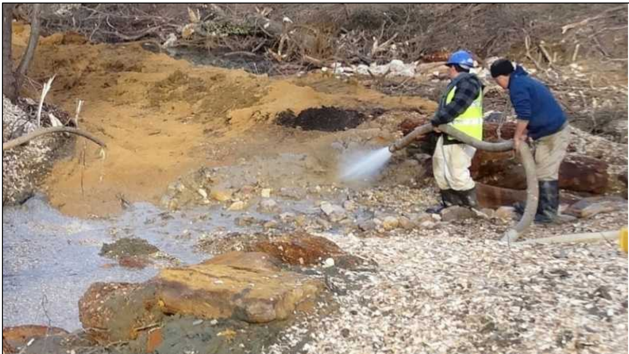
Figure 41. Wash in structures with sand and gravel to fill voids. This should be repeated to sufficiently fill voids, observe flow paths and adjust, if necessary, with more gravel and cobble.
