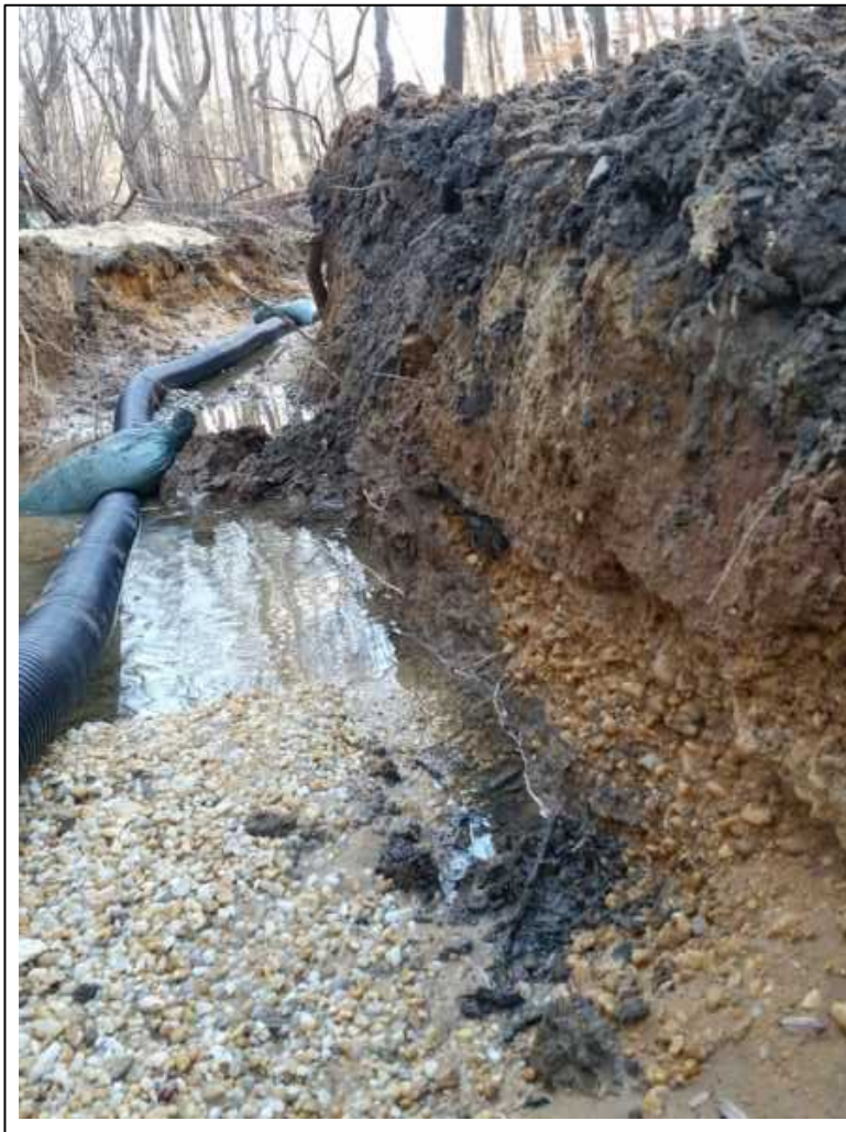
Figure 29. Installation of pea gravel under-drain and seam starting to connect to the native gravel seam (darker gravel on the right side of photo beneath the layer of soil) that has been broken and exposed by bank erosion.
