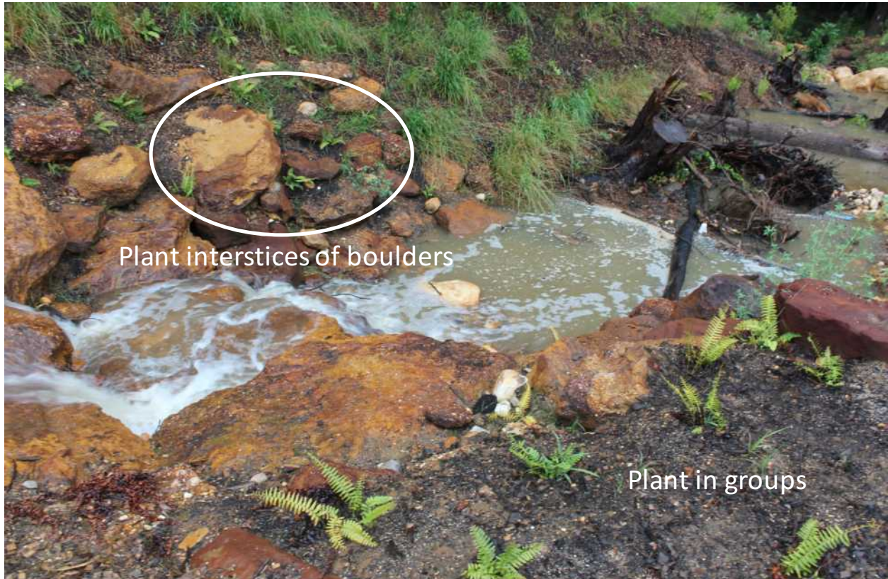
Figure 60. Plant herbaceous in crevices of boulders and group plants rather than uniform lines.
