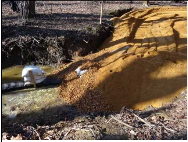
Figure 24. Placement of pea gravel seam over secured slotted pipe and construction of sand and woodchip haul road over the underdrain.
