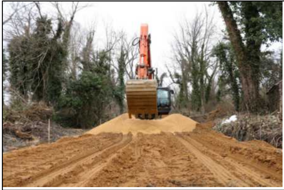
Figure 17. Construction of in stream haul road with sand and woodchip. Contractor backs trucks to the edge, as evidenced by tire tracks, and dumps material in place.
