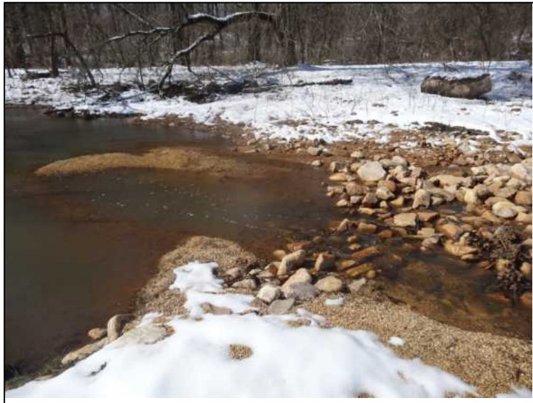
Figure 32. “Cobble weir” with footer boulders submerged and river rocks (cobble) used to hold the grade. It was constructed with sufficient gravel in pools, riffle-weir and along edges to enable formation of diverse flow characteristics, stream bed and habitat.
