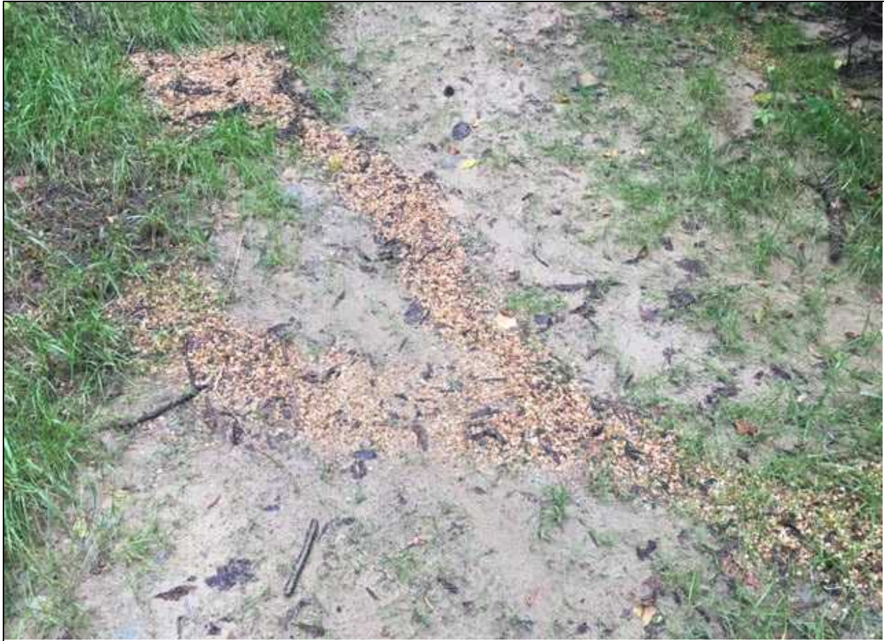
Figure 57. Rills filled to grade with pea gravel to allow water flow to continue in the path it has carved into the newly constructed landscape.
