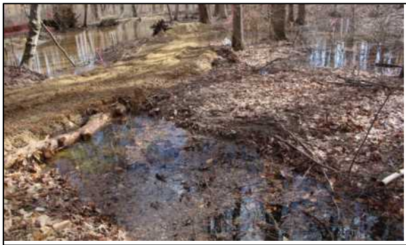
Figure 13. During haul road construction along the edge of the stream, this contractor minimized the width, avoided tree removal and preserved the existing depression on the floodplain (wet areas at the bottom and right side of the photo). Clean sand was used to bridge the haul road across the depression to allow drainage and the depression was not filled or levelled to preserve a diverse topography. Logs were used to keep sand from spilling into the depression, which was kept intact throughout and post construction as seen in the next figure.
