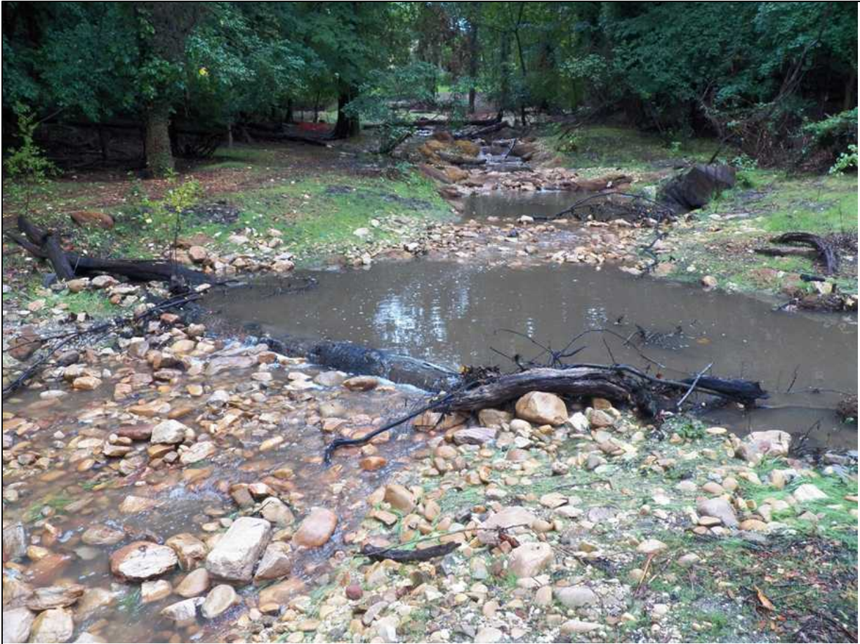
Figure 54. A pool that was widened to further dissipate energy. Edges supplemented with gravel and river rock to create roughness, support diverse geomorphology and provide habitat.
