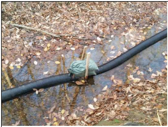
Figure 23. Slotted pipes must be secured with sand bags and stakes to prevent buckling during pea gravel seam installation.
