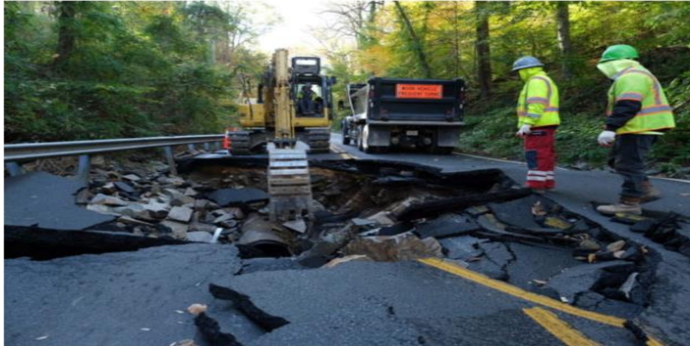
13. Sinkhole caused by large water main break (staff photo by Jay Westcott)
